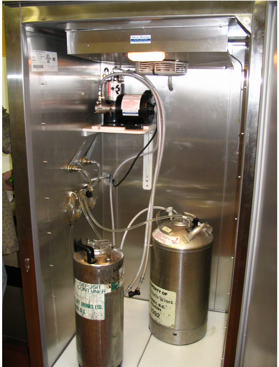
IB 200 Interior View – Left Side
